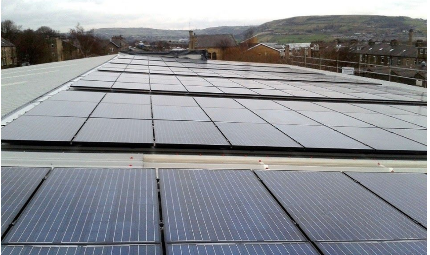
Solar panels on roof of CAIR building
